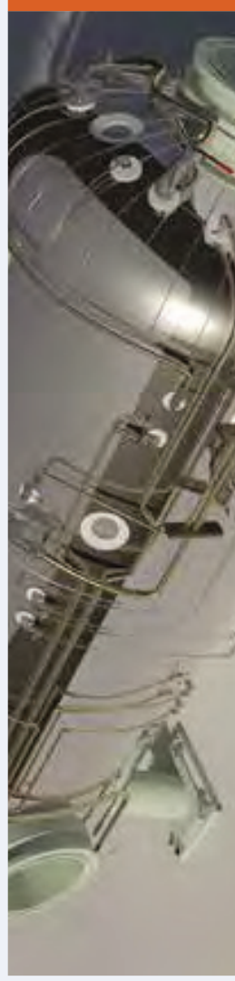
Fig 1. Tungum Tubing installed on a saturation diving system module.
